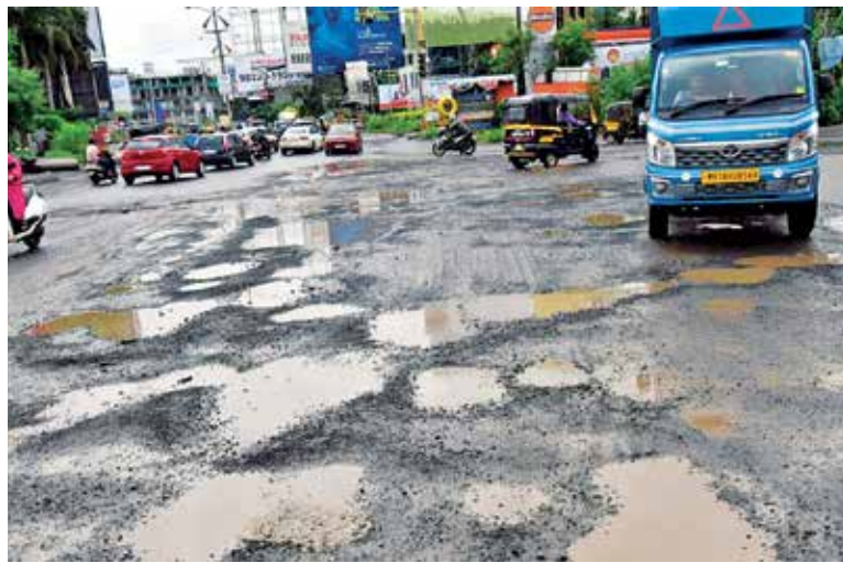
Potholed roads turn into rivers
